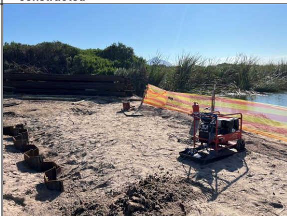
PHOTO 24: Generator on site with drip tray
