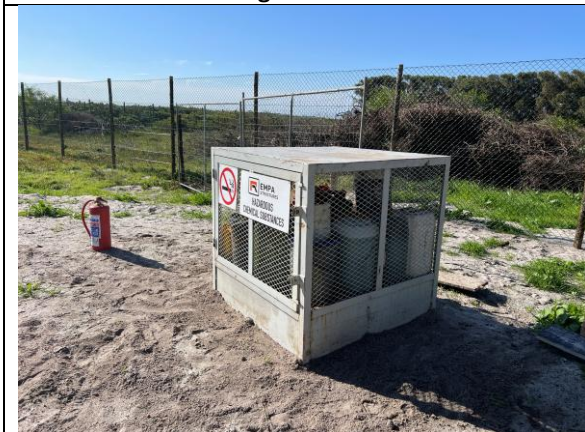
PHOTO 21: Hazardous chemical substances locker (bunded)
