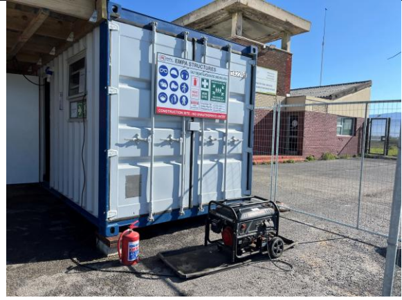
PHOTO 2: Site office – generator, drip tray and fire extinguisher
