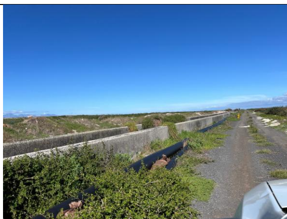
PHOTO 12: Pipelines – dredging line and return dewatering line (to WWTW)
