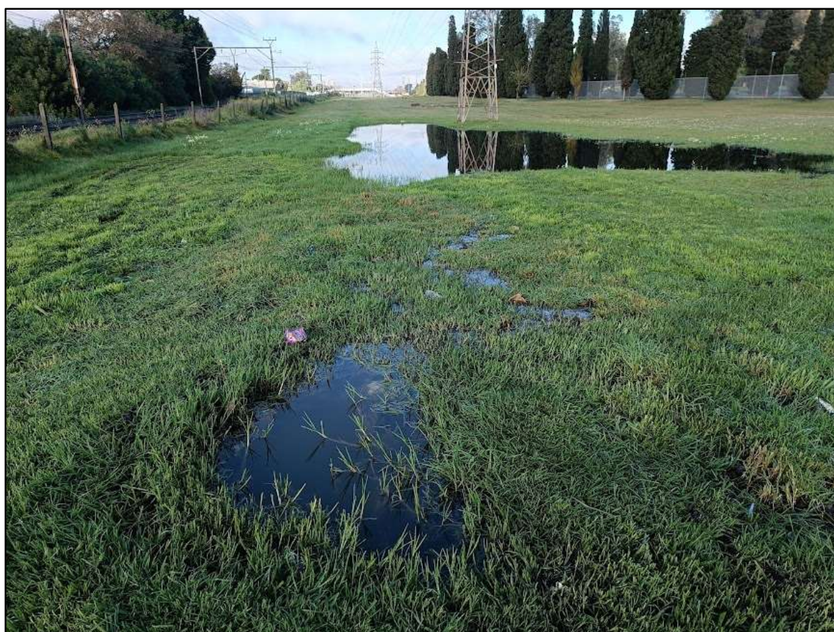
Figure 15: Ponding visible in the area near the overflowing stormwater manhole.
