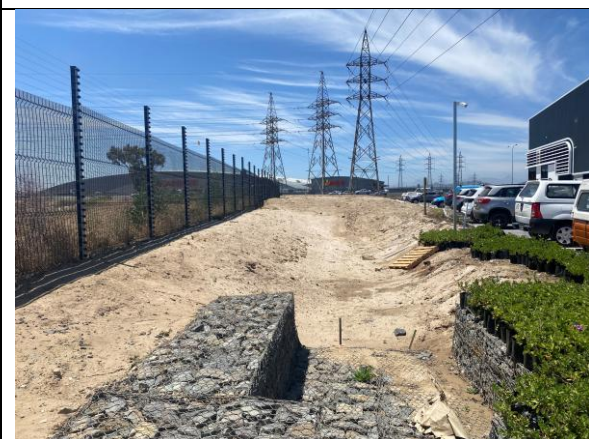
PHOTO 5: Stormwater attenuation facility north of the site (note that this has been seeded with veld grass, which still needs to establish – this must be monitored to ensure successful establishment and ongoing stability of the area).
