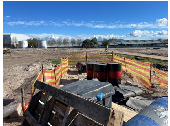
PHOTO 8: Tack drums in a designated area but no soil protection and not in a bunded area
