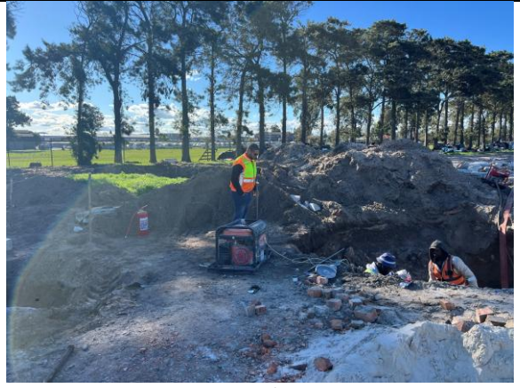
PHOTO 16: Good use of drip trays under generator and pump
