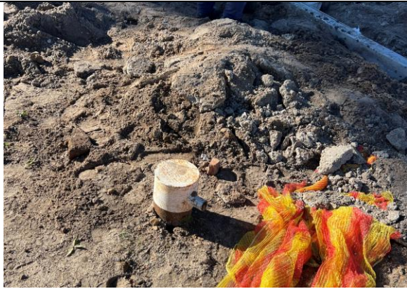
PHOTO 19: Capped monitoring borehole (MW3)
