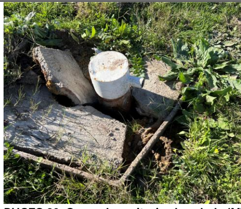
PHOTO 20: Capped monitoring borehole (MW1) but the concrete cover is damaged and requires repair
