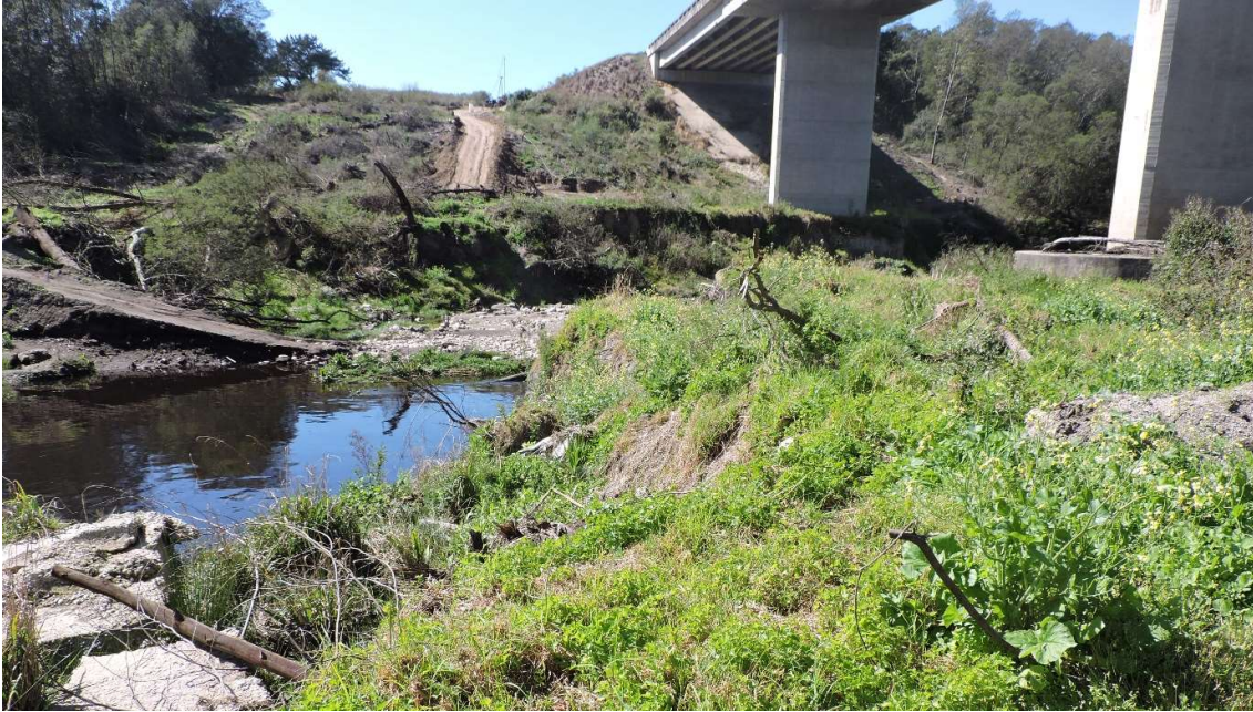
Figure A8: View of the northern (upstream) side of the bridge. Note the existing disturbance of the river bed and banks.
