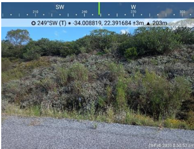
Photograph 12: Showing establishment of indigenous plant species in places along side slopes west of the bridge
