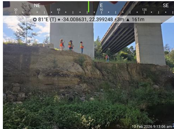
Photograph 19: Showing eroded eastern bank
