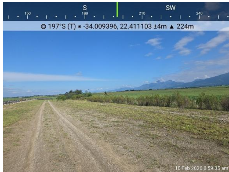
Photograph 11: Showing the eastern side completed to subgrade level and grass and weeds sprouting
