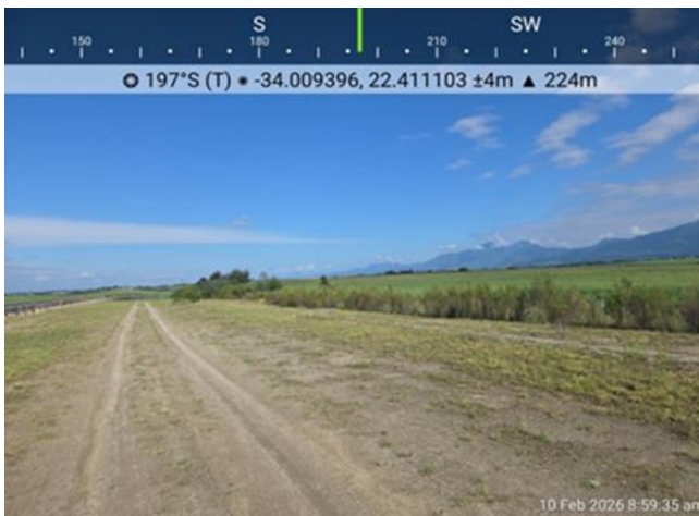
Photograph 16: Showing the eastern approach road alignment resprouting grasses and weeds completed up to subgrade level
