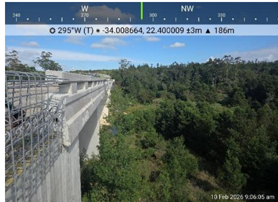
Photograph 2: Showing the top view of the end point of the two completed spans
