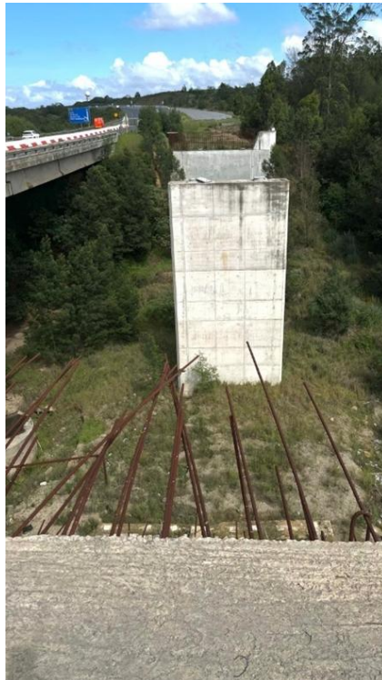
Photograph 8: Showing the top view of the missing western spans of the bridge
