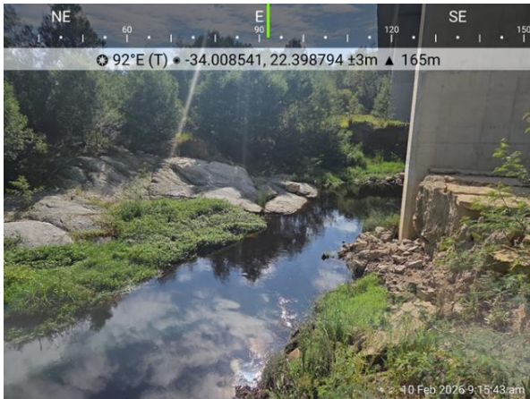
Photograph 18: Showing eroded fill material around the pier
