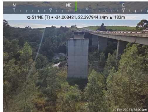
Photograph 4: showing a full constructed pier and outstanding two western spans to be constructed.
