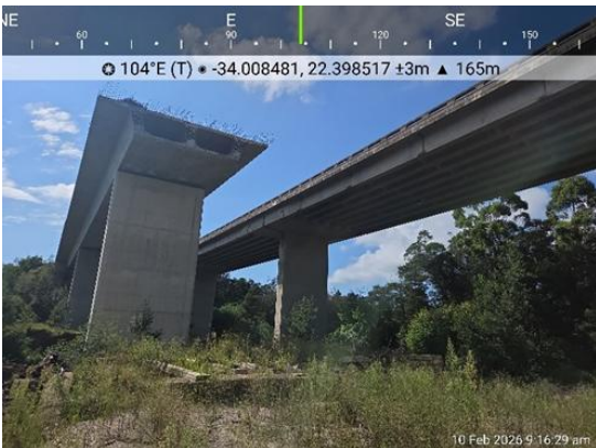
Photograph 3: Showing bottom view of the end point of the two completed spans
