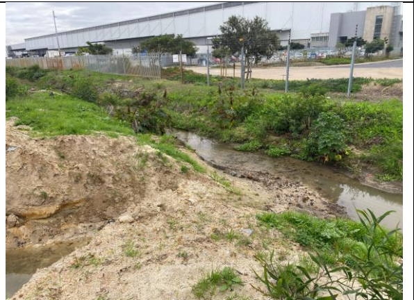
PHOTO 18: Eroded bank of the Duikersvlei in the location of the burst water main – will be repaired after pipe repair and seeded with stabilising vegetation
