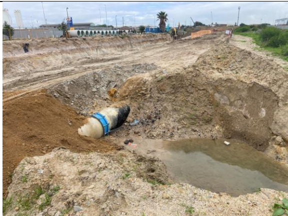
PHOTO 17: Damaged water main in the buffer zone that caused erosion on the bank of the Duikersvlei – awaiting imported parts for full repair
