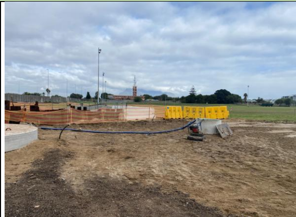
PHOTO 23: Work area demarcation at Theo Marias sports field and ground water dewatering in progress
