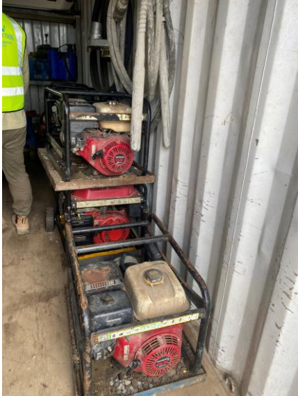
PHOTO 19: Portable generators fitted with built-in drip trays
