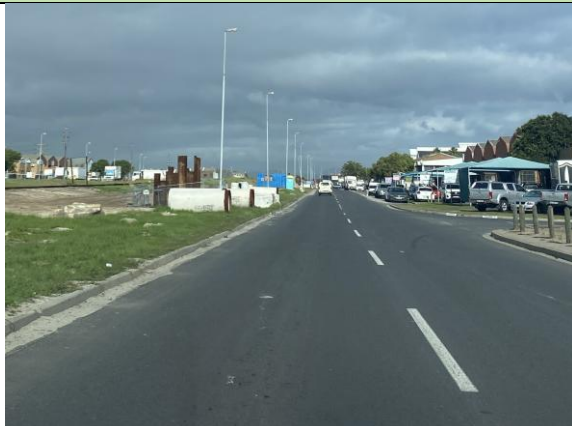
PHOTO 22: Work area along Railway Road – sheet piled launch pit and site toilet provided at key location
