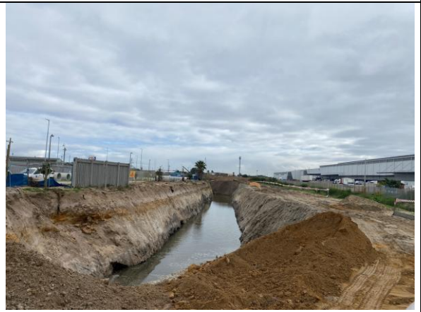
PHOTO 16: Open excavation for sewer line adjacent to Duikersvlei where planned micro-tunnelling is not possible
