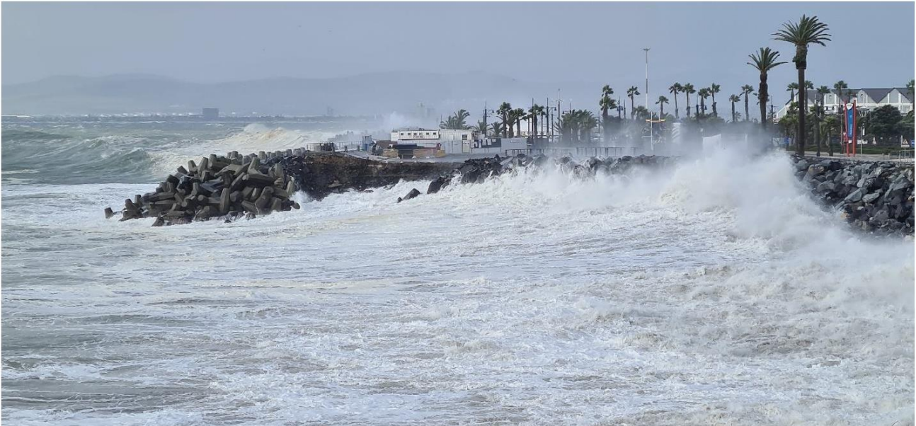
Photograph 0-1. Overtopping of rock revetment at approximately 15:00 on 13 July 2020. Photo credit: Stephen Luger. PRDW, 2025 - extracted from the PRDW Wave and Hydrodynamic Modelling Study.
