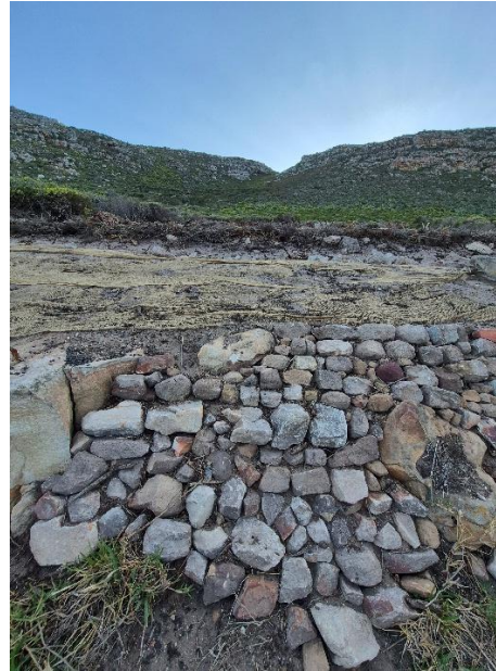
Photograph 11: Loose rocks stacked alongside the M65
