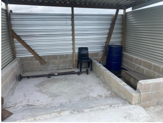
PHOTO 1: Bunded and covered area for parking of diesel bowser and liquid hazmat drums
